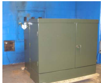
Figure 1 - Pad Mounted Transformer
