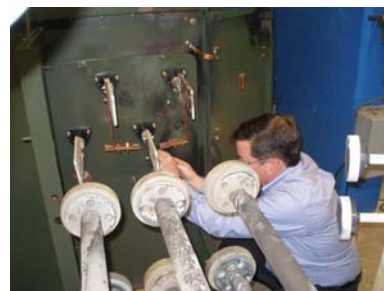
Jim, in the high power lab setting up an arc flash test on a pad mount transformer.
